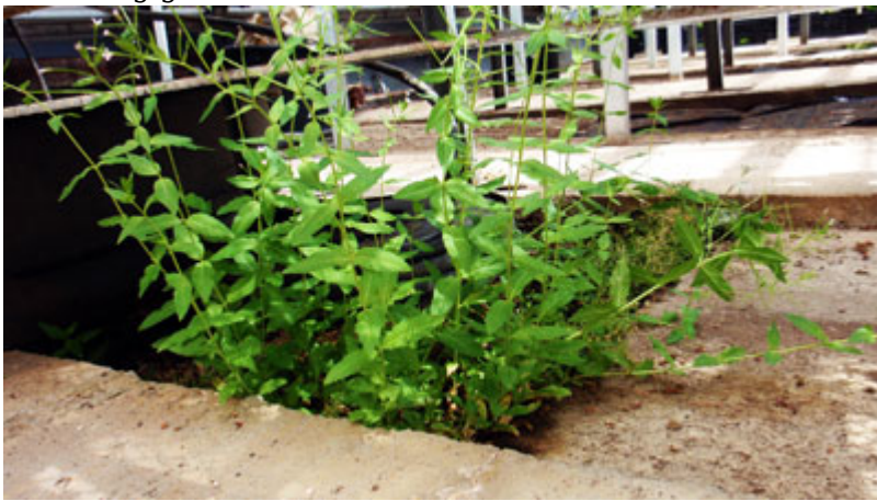
weeds growing inside a greenhouse
